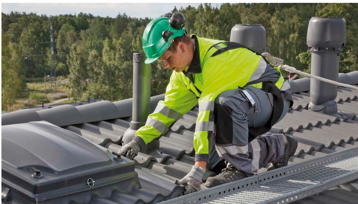
KerabitPro is a leading roof installer in Finland and works with all types of roofs. In addition to installing, maintenance and renovation are an important part of the service offering.
