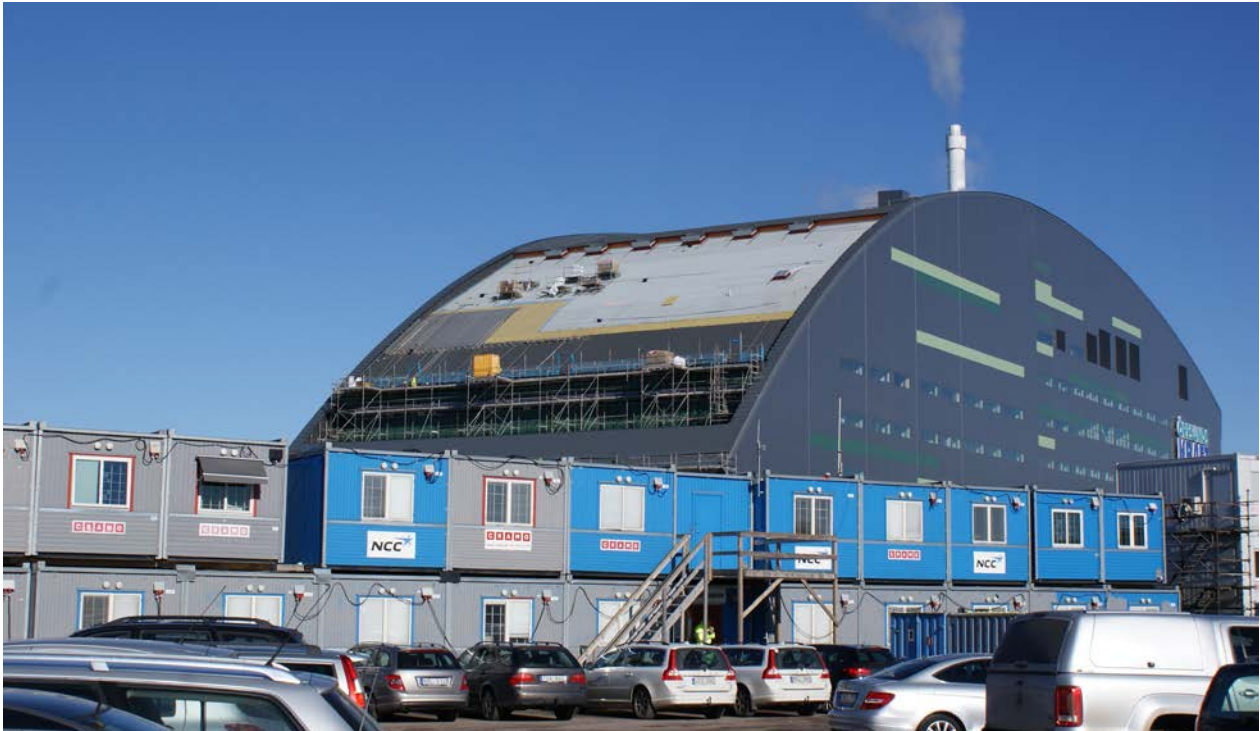
The roof of Filborna combined power and heating plant in Helsingborg was covered with 9,000 square meters of waterproofing from Matak.
