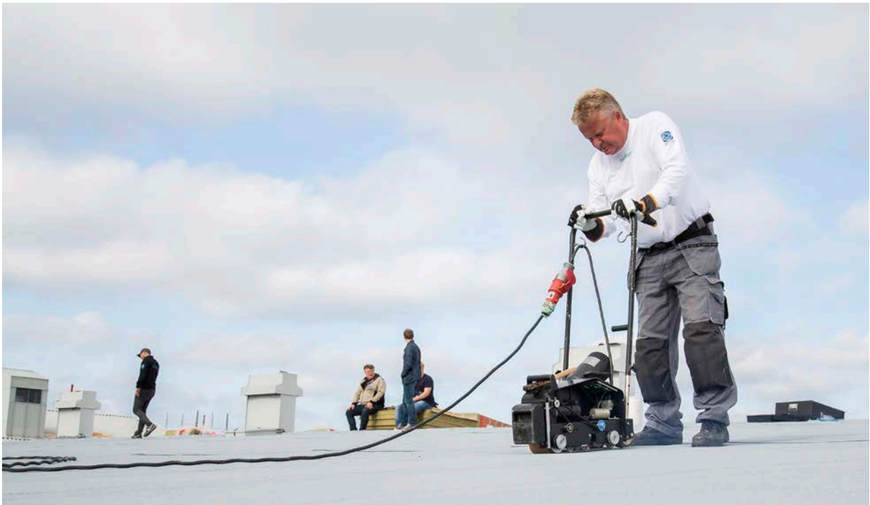
Installation of Matakì UnoTech® FR LESSNOX, a bitumen based waterproofing coated with a slate of titanium dioxide. In combination with UV light nitrogen oxides from pollutions are converted to nitrate, which can be taken up by plants.
